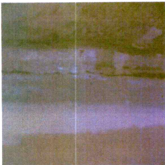
Picture is of the interior of the tank where leak was discovered.
